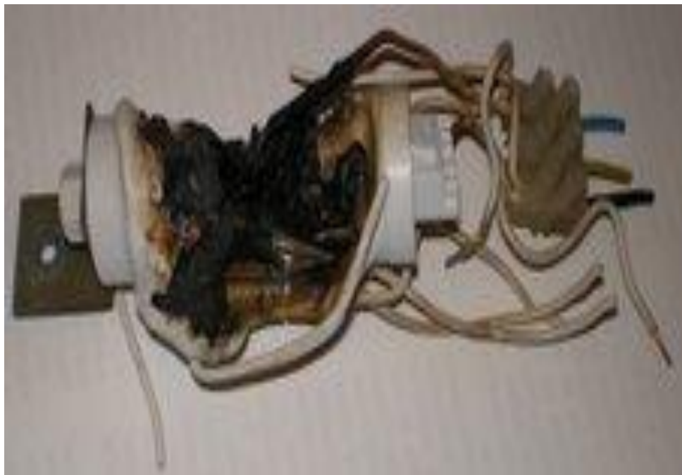
Figure 7: Compensation capacitor damaged due to defect
