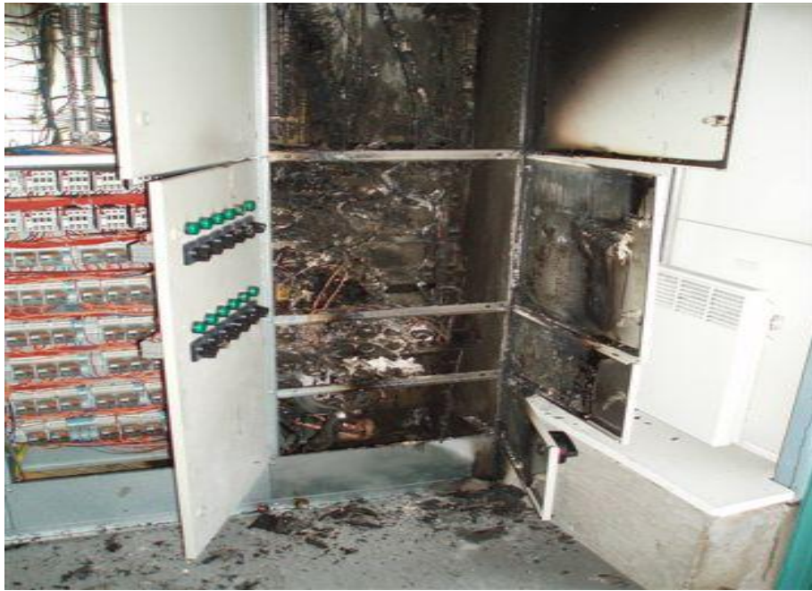
Figure 4: Installation box destroyed due to loose connections or a worn component
