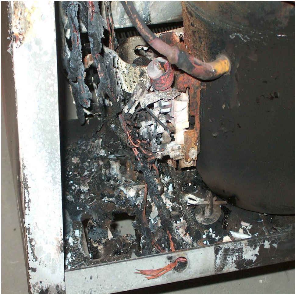
Figure 6: Fire-damaged refrigeration equipment
