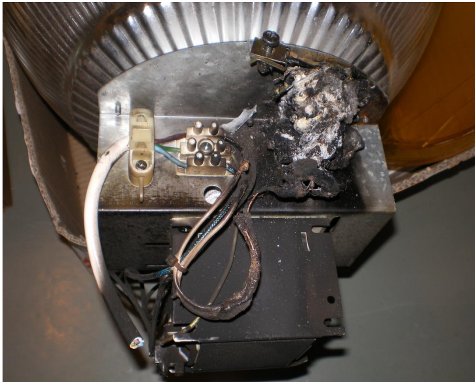
Figure 5: Floodlight damaged due to defect in compensation capacitor
