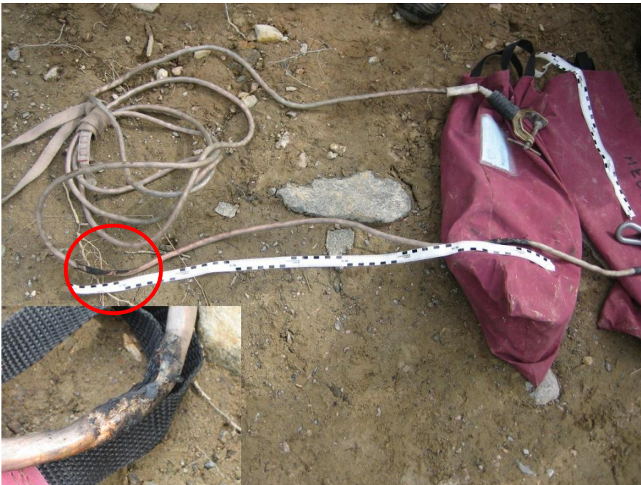
Figure 6. The temporary earthing device used in the work leading to the accident.
