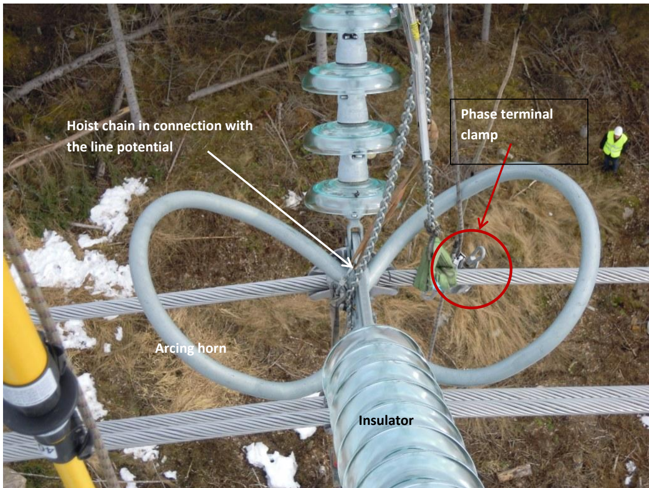
Figure 5. The site after the accident, 18 April 2013.
